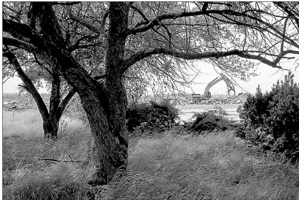
A trackhoe takes prey Tuesday on what used to be, the truck plant at Opdyke and South Blvd.
